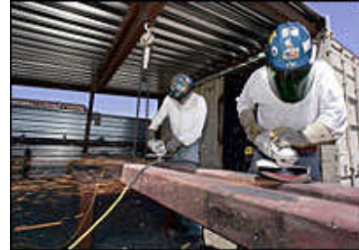
Ironworkers Brian Plotezka, left, and Craig Humphries clean up a beam at the Schuff Steel Co. yard on Tuesday. The beam will be used in a temporary staircase during construction of the Palazzo.
